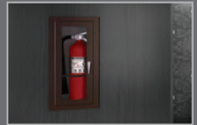
FIRE CABINETS + EXTINGUISHERS
