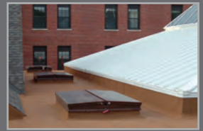
ROOF HATCH + SMOKE VENT
